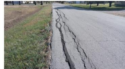
Cause is shrinkage of clay subgrade due to loss of moisture.
