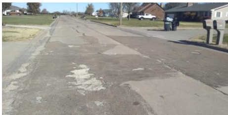
Heather was constructed in 1996 and has had issues for quite a number of years.
